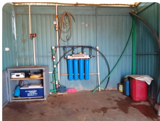
Inside the kiosk: the filtration line, with pump, battery and control unit to the left.
