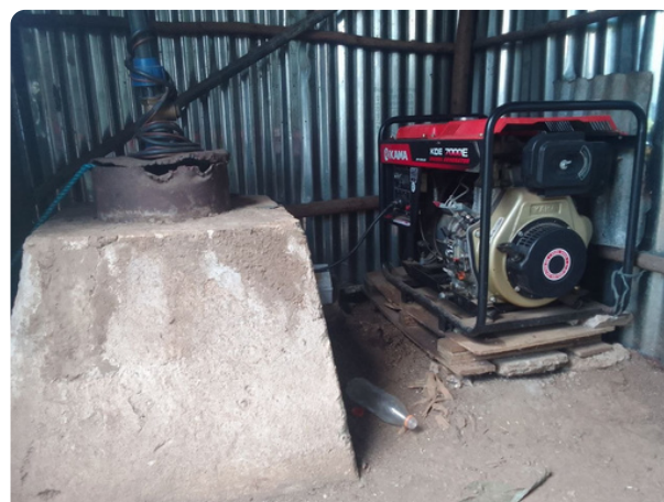
The diesel generator that drives the kiosk pump. Fuel was the single largest operating cost, and its unavailability — not its price — is what eventually stopped the business.
